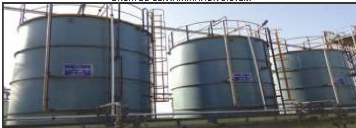
EFFLUENT STORAGE TANK
